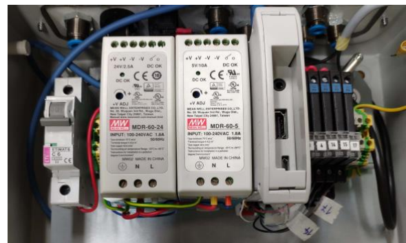
Figure 3: The main components of the ROS peripheral interface from left to right: safety fuse, power converters (24V and 5V), micro-computer and relays.
